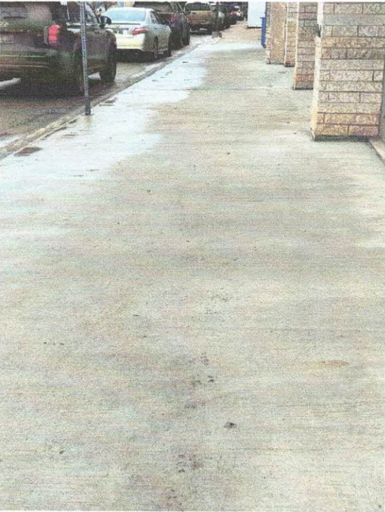
Replacement of sidewalks remains to be a priority!
